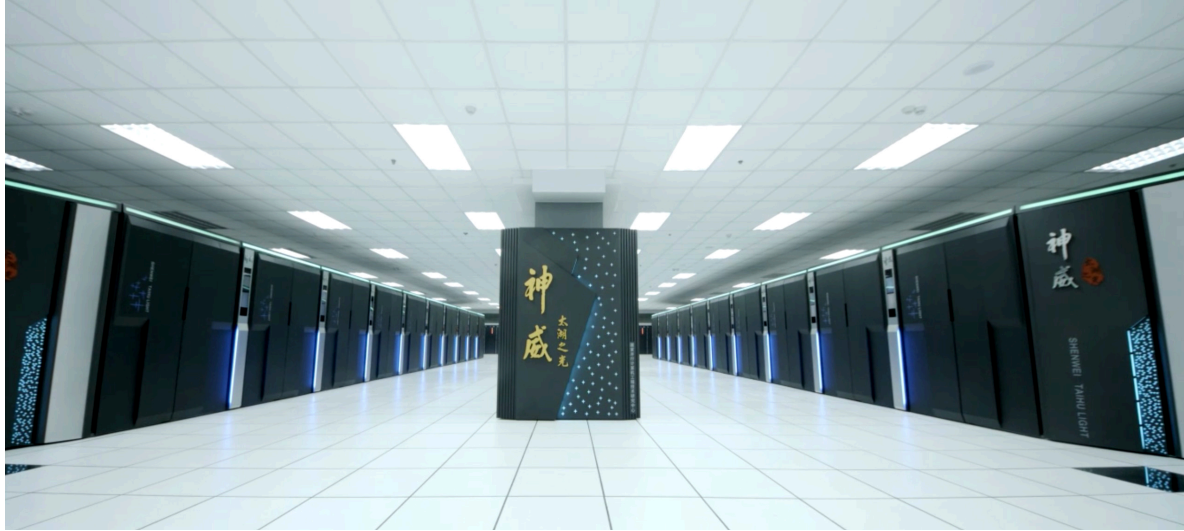
Figure 5: Picture of the Sunway TaihuLight System computer room
